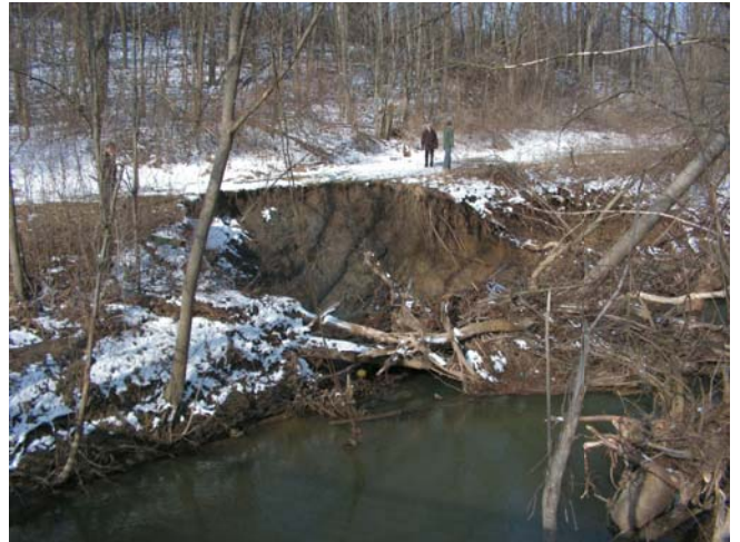
Severe erosion on the Black River
